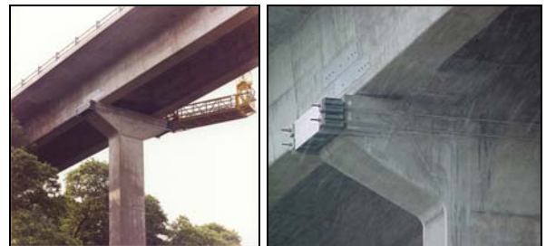
High level stressing work was executed without a single lost time incident
