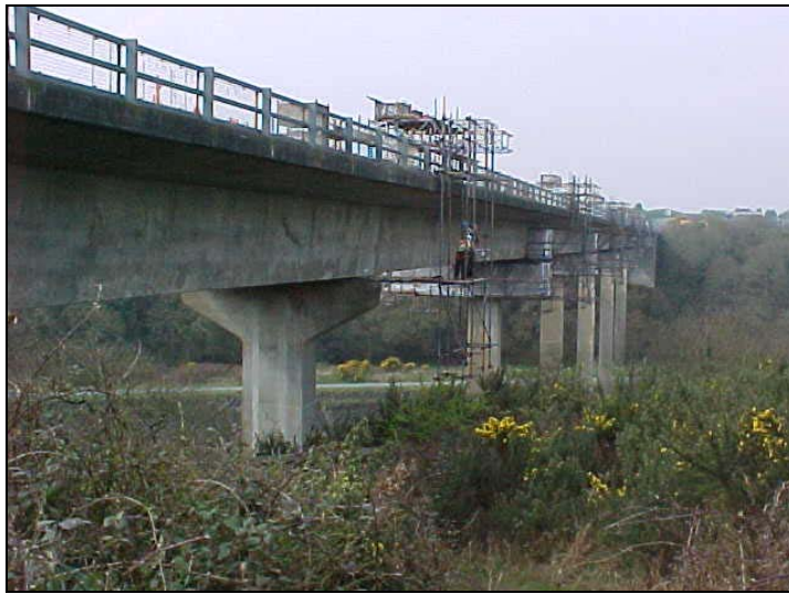
Westfield Pill Bridge carries the A477 over the Milford Haven basin the cross heads
