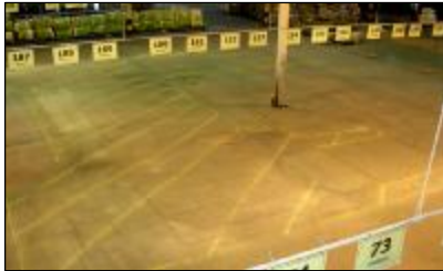
Failed concrete was identified & replaced
