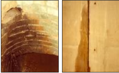
Brickwork and joints are prone to leak ...
