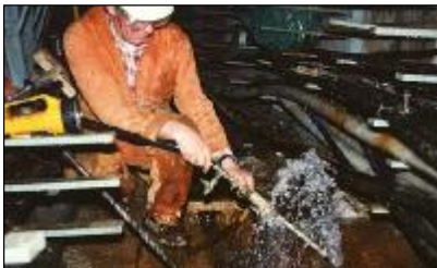
Leakage can disrupt services if untreated
