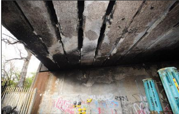
Damage caused by Fire
