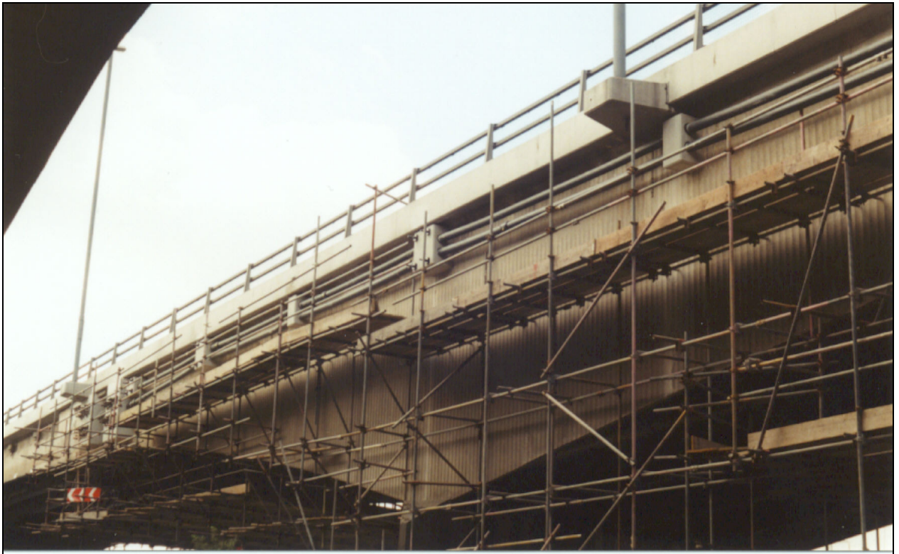
Clifton Bridge carries the A52 over the River Trent near Nottingham. The two bridges each carry one carriageway of three lane traffic.
