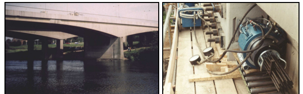
42km of tendon were installed in the box sections of the bridge
