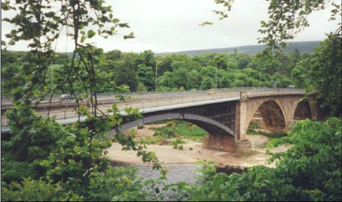
The bridge spans the River Spey, which is a Class 1 Watercourse and important salmon fishing river.
