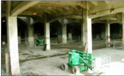
The warehouse was in a decrepit condition
