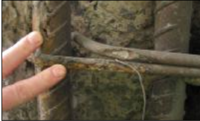
Chloride attack evident on link rebar
