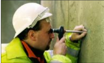
Diagnostics and testing was undertaken
