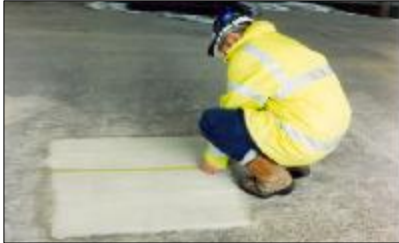
Major concrete repairs were needed
