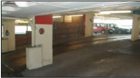
The car park suffered from disrepair
