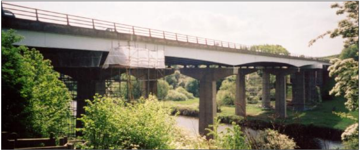
Heavy bearing installation at height and adjacent a river were some of the challenges facing the contract team
